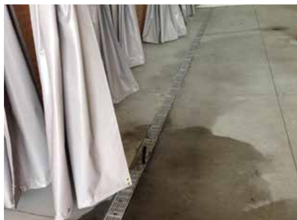
Fig. 3 b: Decontamination Shower Trench Drain
